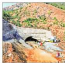
The final breakthrough of the 1.5-km-long tunnel of the bullet train project in Palghar.
