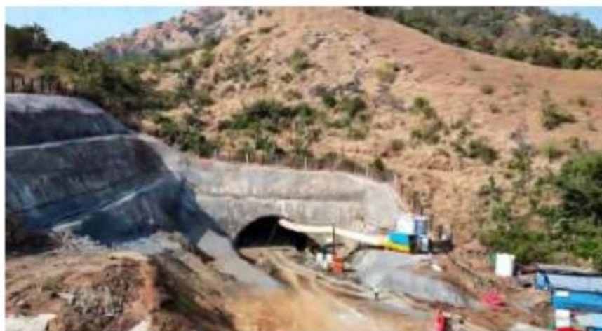
The first breakthrough of a 1.5-km-long mountain tunnel of the bullet train project in Maharashtra's Palghar district. PTI
