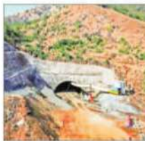
The final breakthrough of the 1.5-km-long tunnel of the bullet train project in Palghar. PTI
