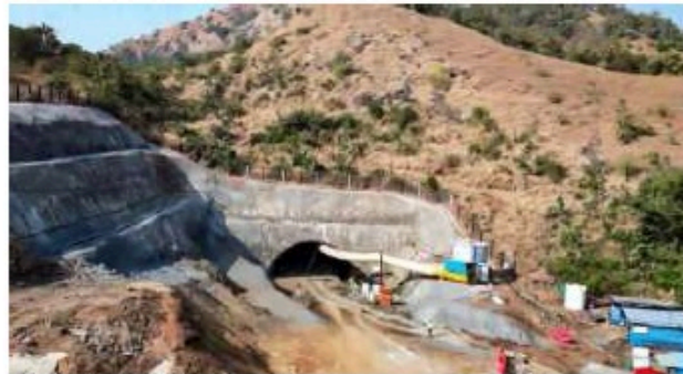
The 1.5-km tunnel is the longest among the seven planned in Maharashtra for the bullet train corridor. PTI
