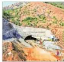
The final breakthrough of the 1.5-km-long tunnel of the bullet train project in Palghar. #1
